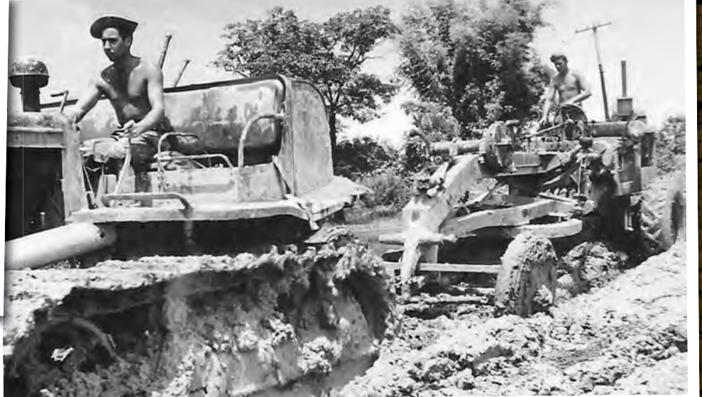
Above: International TD 18 pulling a scraper at work between Makum Junction and Digboi, Assam (1880th Aviation Engineer Battalion).
