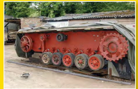
Above: Work started on the lower hull first, with Jon, aided by various friends and other enthusiasts, carrying out the repair work.
