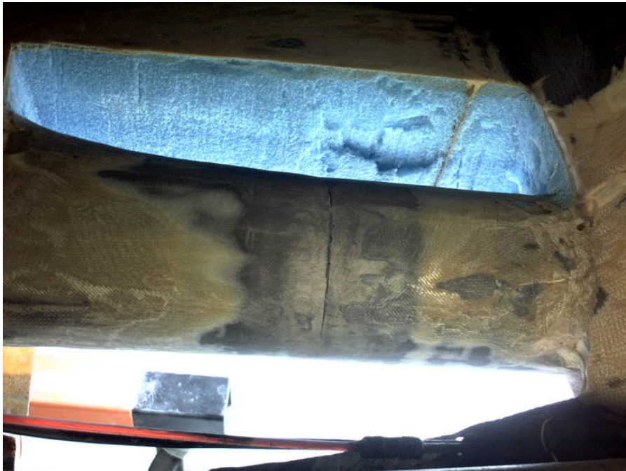
Crack in top of spar
