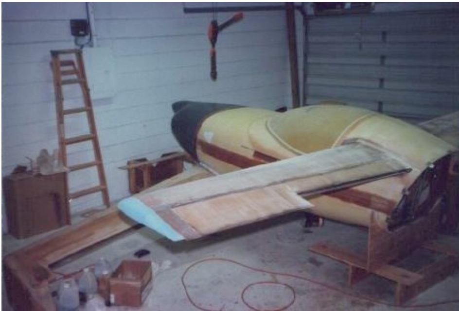
Another view but you can also see work being done on the wing tips.
